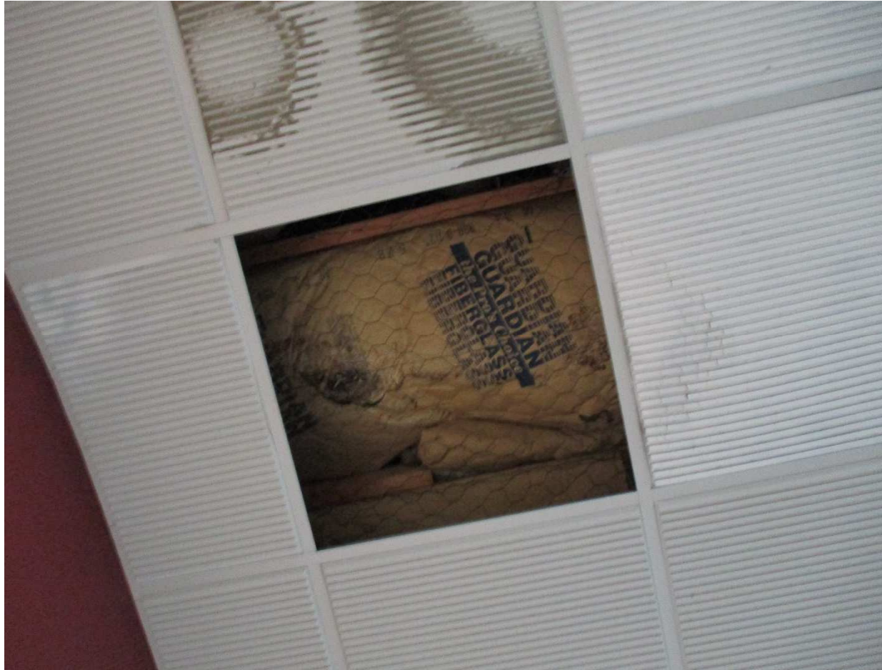
Plenum Insulation Failure
