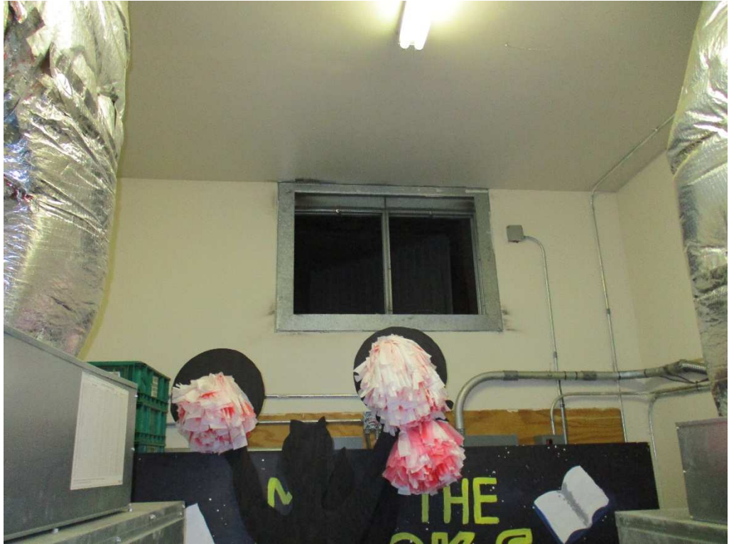
Plenum Return Opening into Mechanical Room
