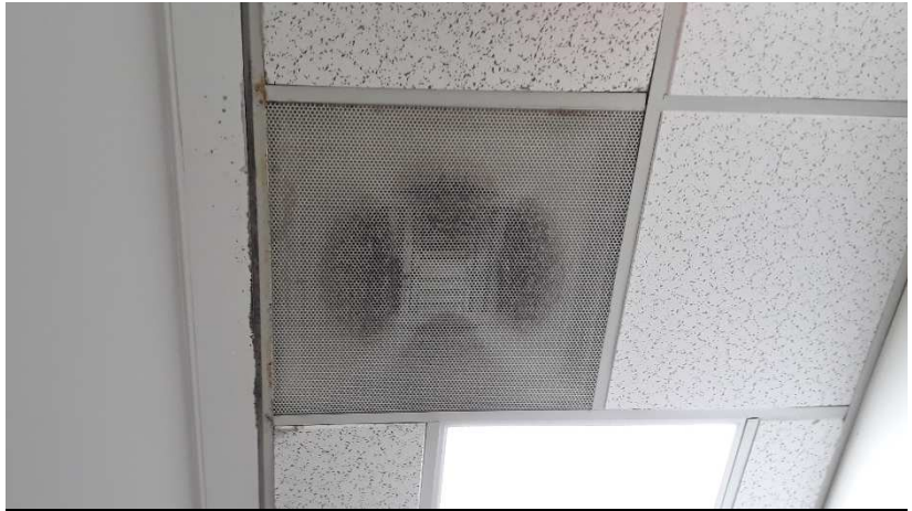
Dirty Ceiling Diffuser
